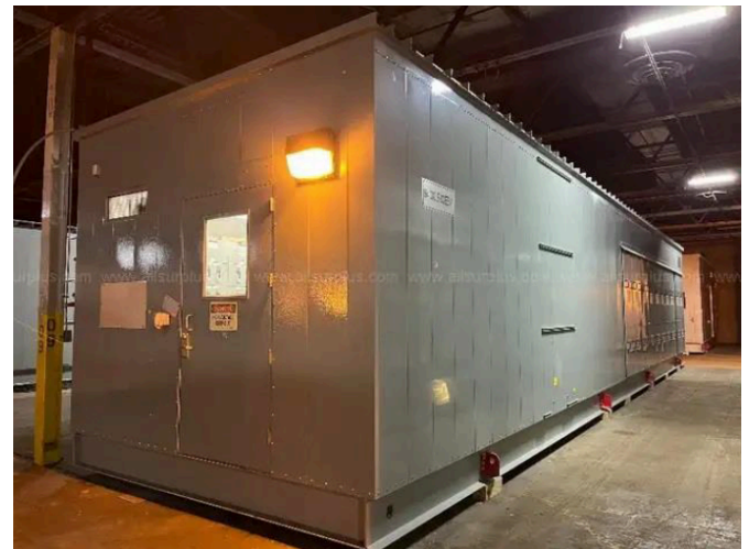
2012 Electrical Equipment Shelter
